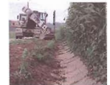
Gradall excavator at work on Gardner, Mobley, and Myers Roads this past summer in preparation for a widening and resurfacing program funded by an OPWC grant.
